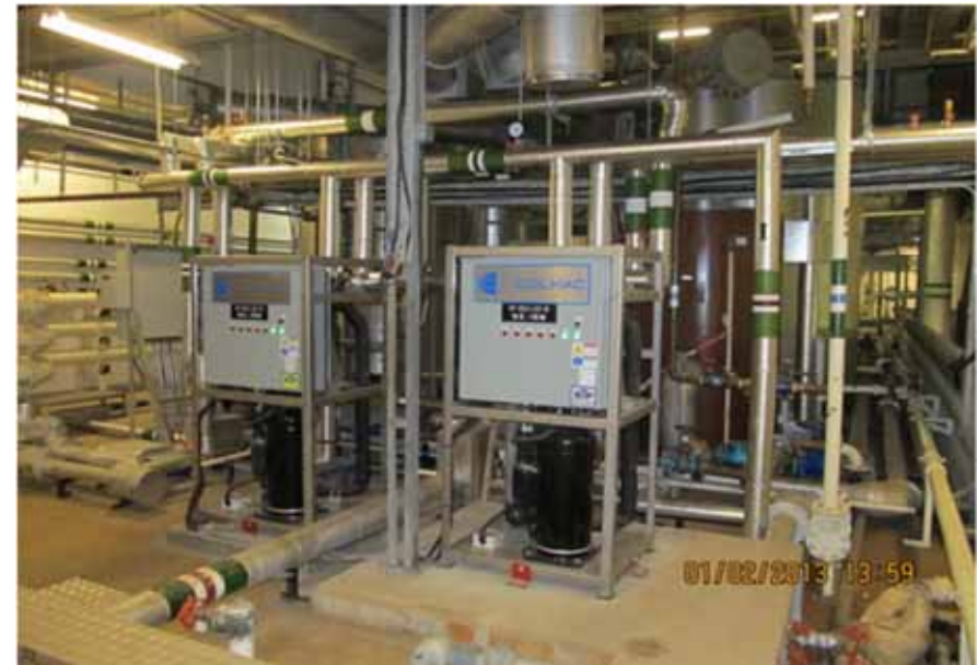
RPT Calculations with Performance Result: Smart Energy System for Waste Heat Recycle From Chiller to Hot Watering 2013
